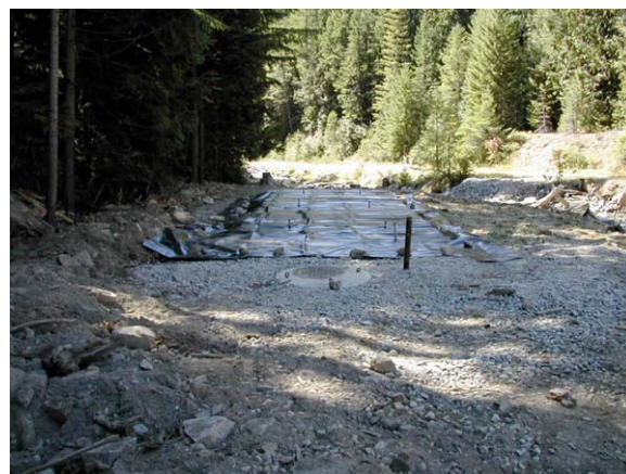
Fig. 4. The emplaced Apatite II PRB at the Success mine, between the East Fork of Ninemile Creek and the tailings pile, September 2002.
