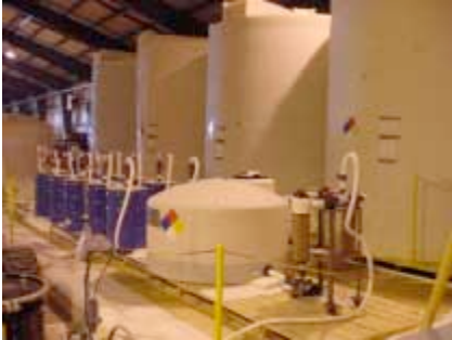
Figure 1. Apatite II Treatment System for U and RCRA Metal Contaminated Wastewater
